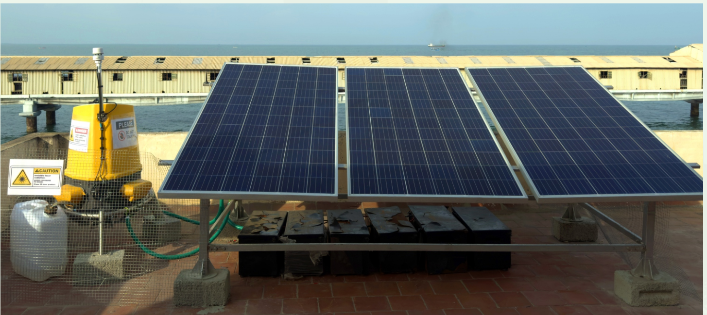
VOC PORT_2, Location: Electrical Substation terrace near oil jetty
