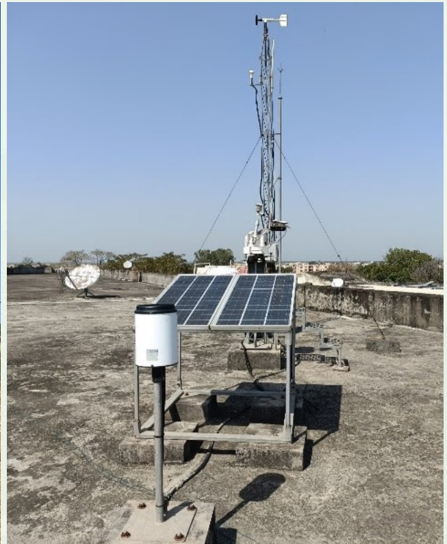
SRRA Station Installed in Madhya Pradesh
