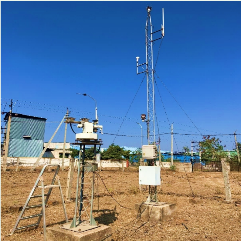
SRRA Station Installed in Karnataka
